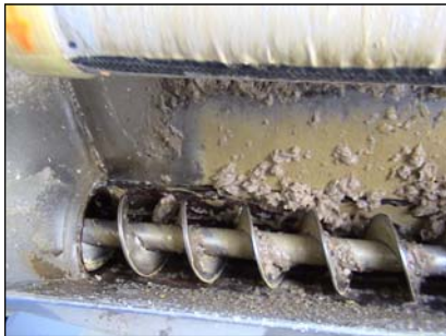
In the hopper, a screw press dewateres the solids to a cake with up to 40% solids.
